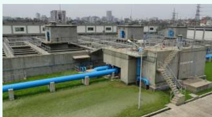
500 MLD Gandharbpur WTP 24km Raw Water Pipeline 15km Transmission Pipeline 21km New Pipe Network ADB- MDSC-DEWSP-DWASA Project
