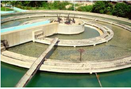
Chandnighat Water Treatment Plant at Dhaka, Bangladesh
